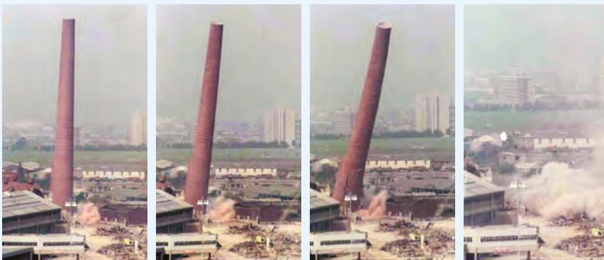
▲ About to go, going, going, gone: last moments of the St Anne's Board Mill chimney
